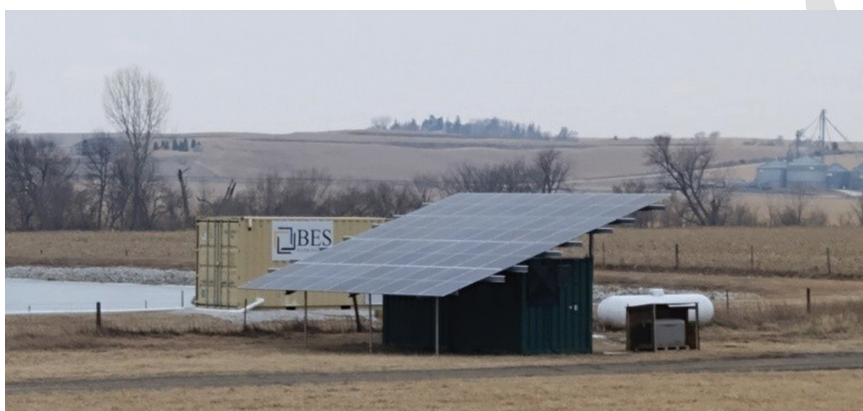
Figure 6. The mobile microgrid supporting a wastewater plant.
