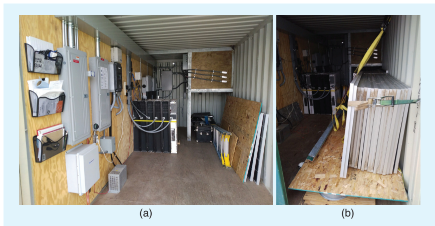
Figure 5. The interior of the container mobile microgrid (a) without solar panels and racking and (b) with solar panels and racking.
