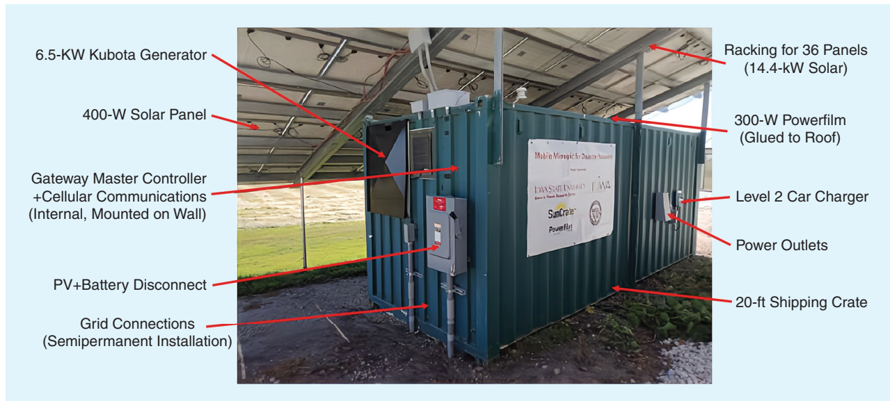
Figure 4. The configuration of the mobile microgrid in a container.
